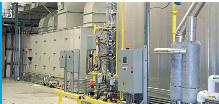
CHP System at Frito Lay facility in Killingly, Connecticut.
